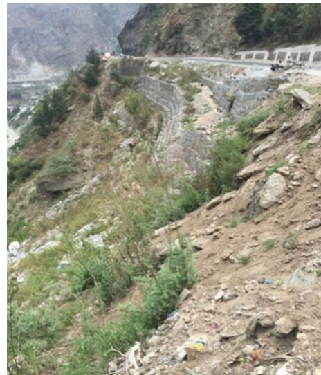
Fig. 1 View of Hill slope showing landslide and movement of soil and gabion wall
