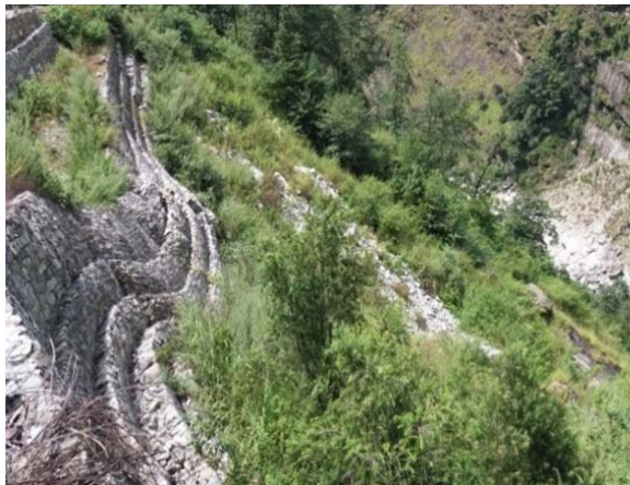
Fig. 6 Displaced Gabion wall
