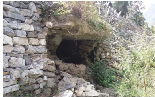
Fig. 7 Damaged Culvert at the valley side
